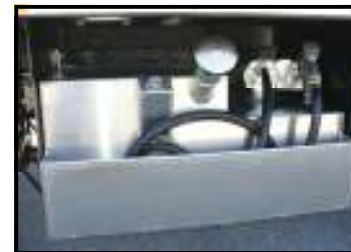
Regular fuel station
