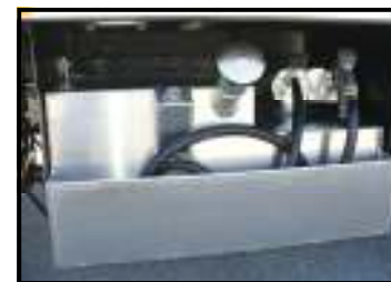
Regular fuel station
