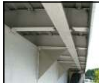
Under deck tie bar
